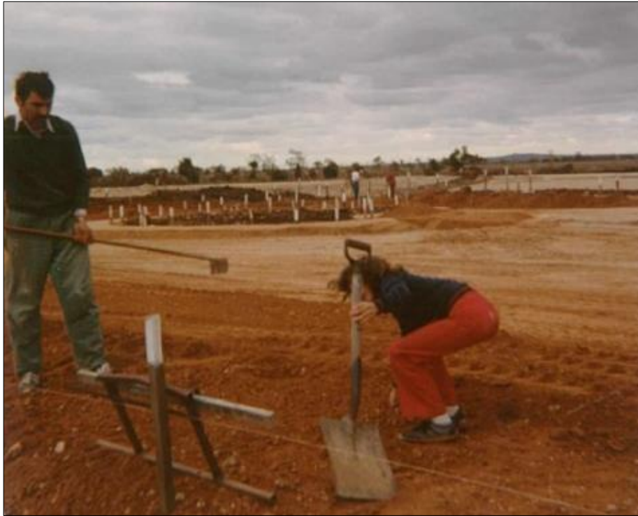
Figure 2: Larissa Kaput (child in foreground) working on the construction at Melton Assembly Hall
